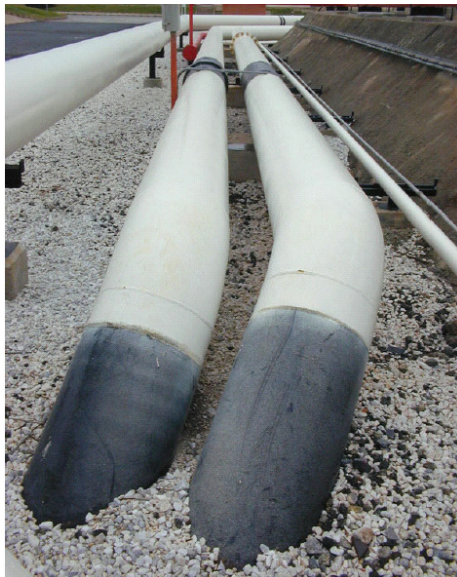
Main hydrant pipes disappearing into the ground
