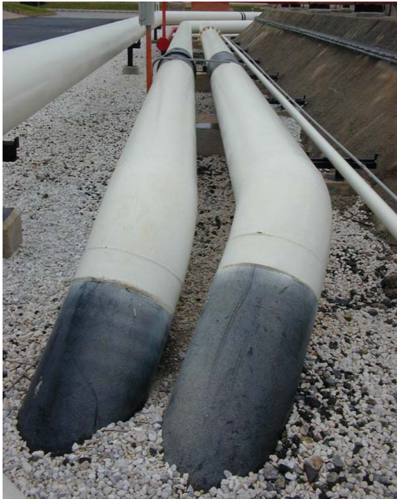
Main hydrant pipes disappearing into the ground
