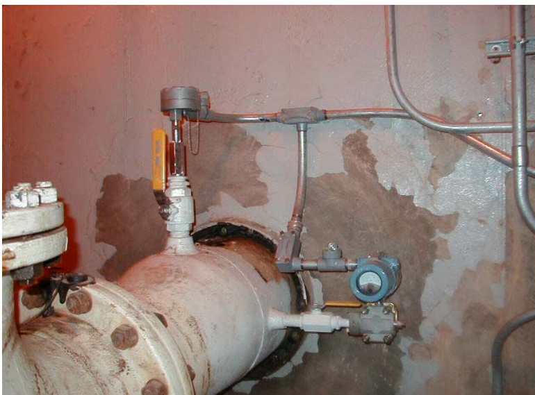
Pressure and Temperature Transmitter on pipe
