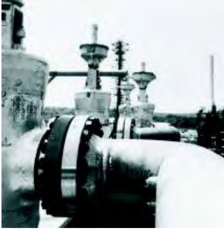
WKM Model D High Temperature Pow-R-Seal Gate Valves in a Synthetic Natural Gas Plant
