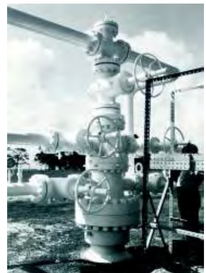
WKM Model E Pow-R-Seal Gate Valves on an LPG storage wellhead
