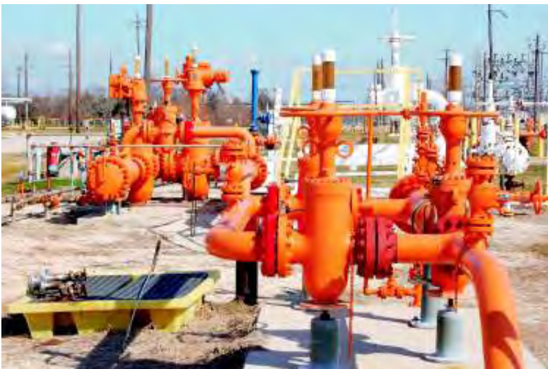
WKM Model E Pow-R-Seal Gate Valves on a gas storage manifold
