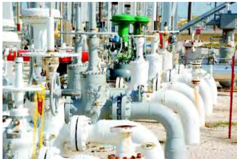
WKM Model E Pow-R-Seal Gate Valve used for switching gasoline and other refined products on a tank farm manifold
