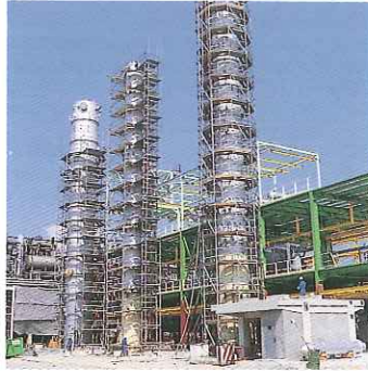
Colonnes (Industrie Chimique). Towers (Chemical Industry).
