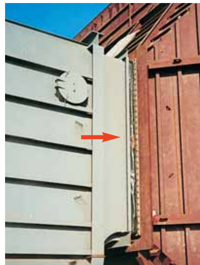
Expansion joint on an electrostatic precipitator in a cement plant
