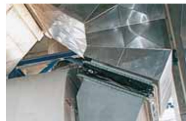
Fan isolation expansion joint
