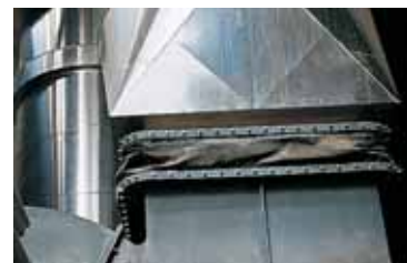
Flue gas duct and expansion joint
