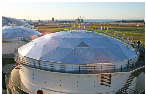
Figure 3. Aluminium dome roofs could provide additional safety features compared to other alternatives including fire protection, protection from unauthorised access, and improved emission controls.
