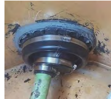
Example of Blueline Large KFD Repaired
