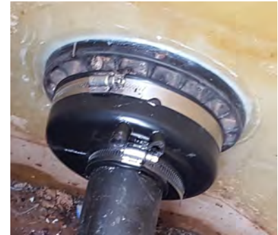
Example of Blueline Medium KFD Repaired
